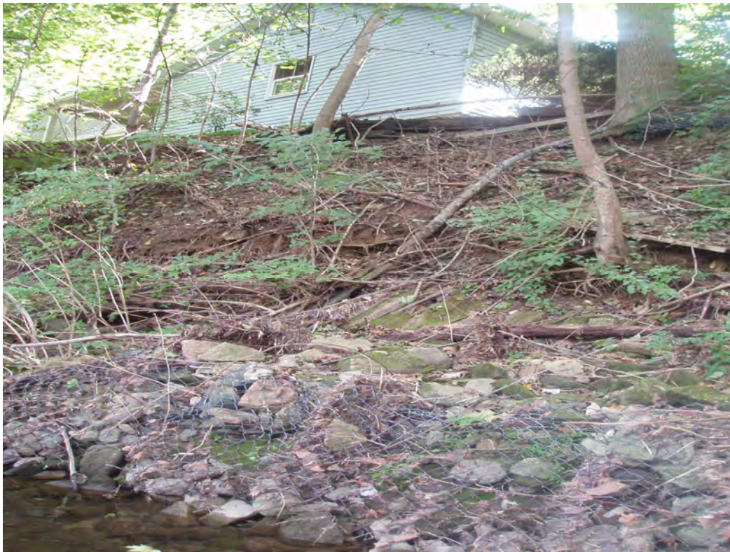
Figure 8. Pre-restoration photo: Bank erosion along the upstream, unrestored reach near the Independence School. Gabion baskets have been installed by homeowners in an attempt to stabilize the banks (Source J. Meyer 2006).
