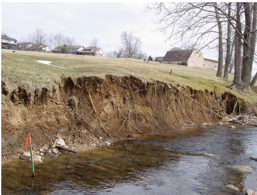
Figure 1. Pre-restoration photo: Severe bank erosion along the Pike Creek mainstem at the Three Little Bakers Golf Course (Source: DNREC 2002)
