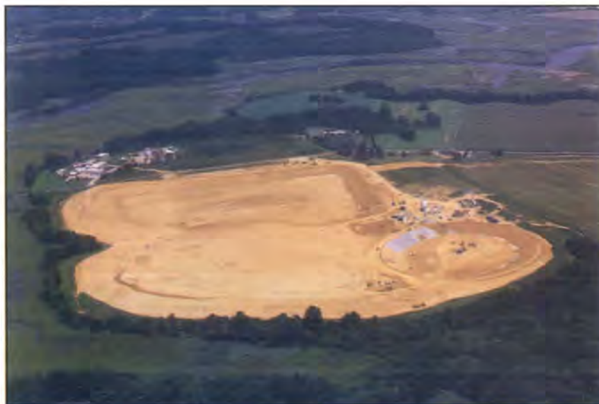
Aerial view of spray irrigation facilities being constructed to treat wastewater in the M-O-T area. Photo by NCC Department of Public Works.
