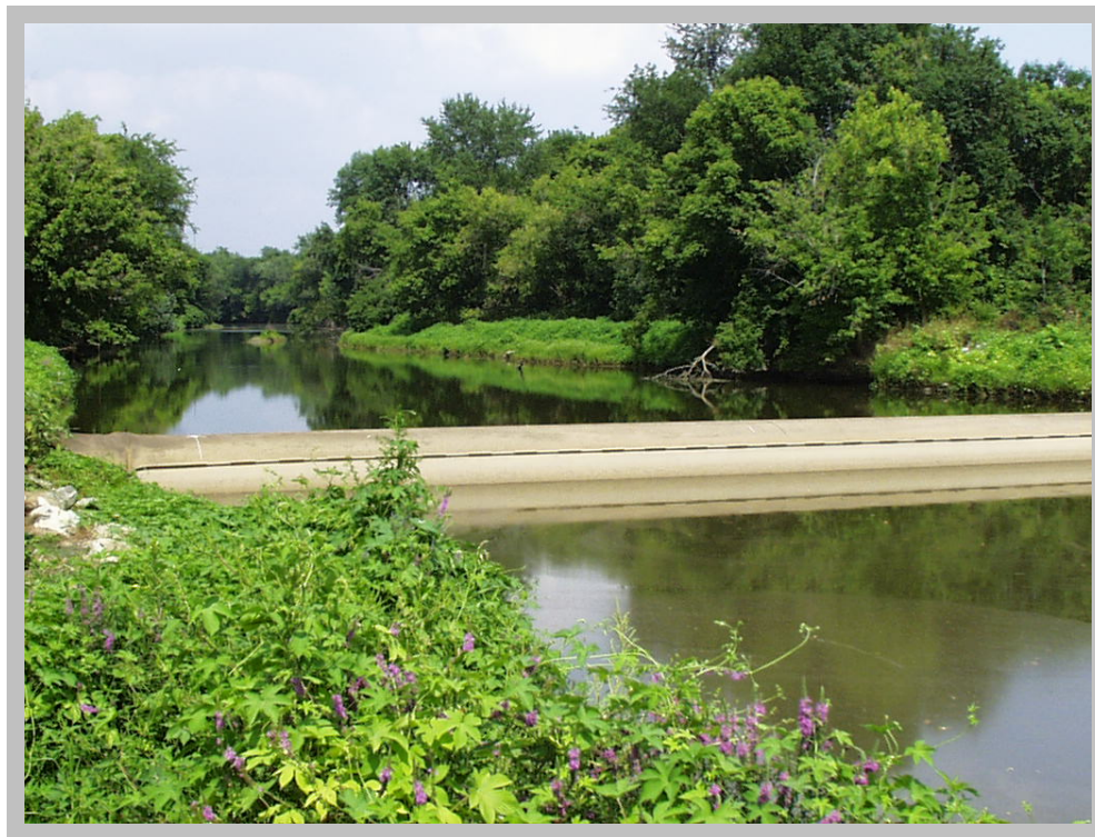
Figure 2. The UWD Tidal Capture Structure along the White Clay Creek at Stanton looking upstream.
