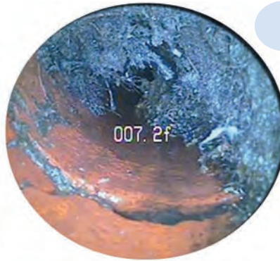
This house has a root problem! This video still shows the cause of the home's plumbing issues.
