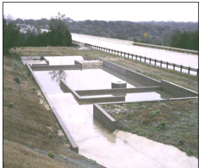
Figure 6: Spill containment should be a feature in highway retrofit designs.
