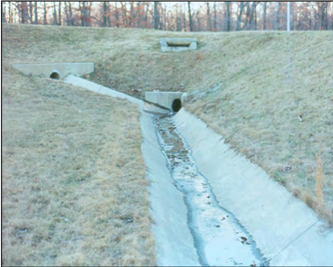
Figure 5: Multiple outlets are a clue that storage trading is a possibility
