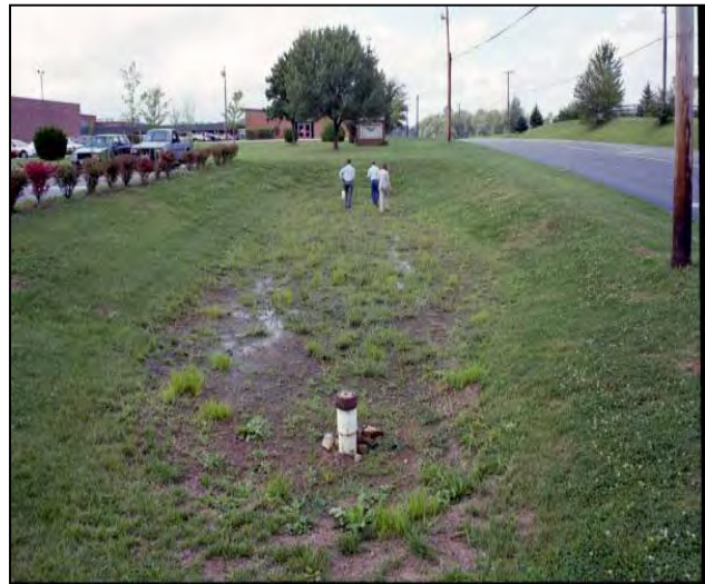
Figure 1: Surface Sand Filter
