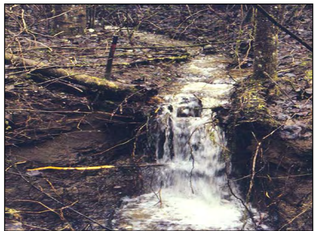
Figure 8: Crews should look downstream for advancing knickpoints that could undermine in-channel treatments.
