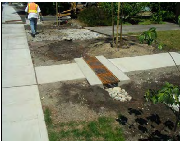
Figure 8: Designers need to find creative ways to pass runoff across driveways and sidewalks.
