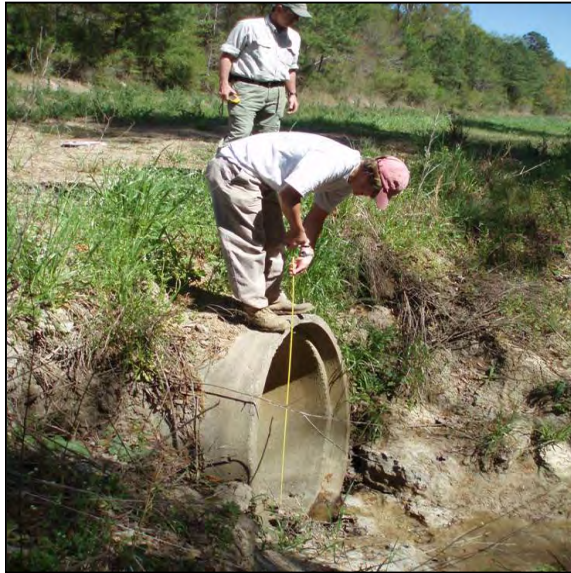
Figure 7: Crews measure the diameter, condition and invert elevation of the storm drain outfall.
