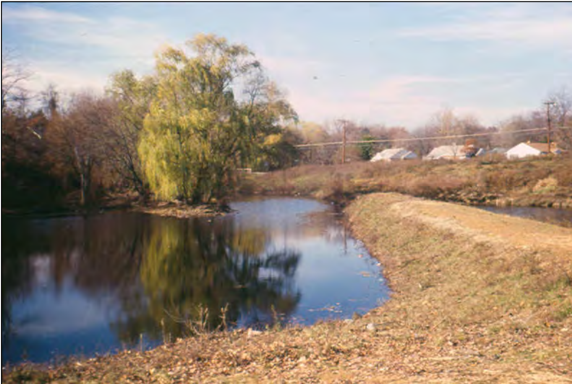
Figure 12: This under-sized forebay filled up with sediment within five years of retrofit construction.
