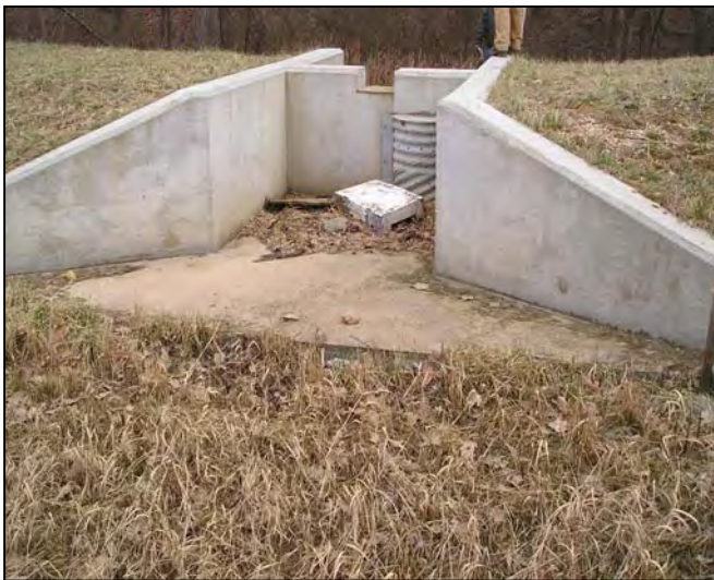
Figure 6: A dry pond retrofit may include the installation of a weir wall
