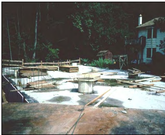
Figure 3: Large underground sand filter under construction to treat runoff near a drinking water intake.
