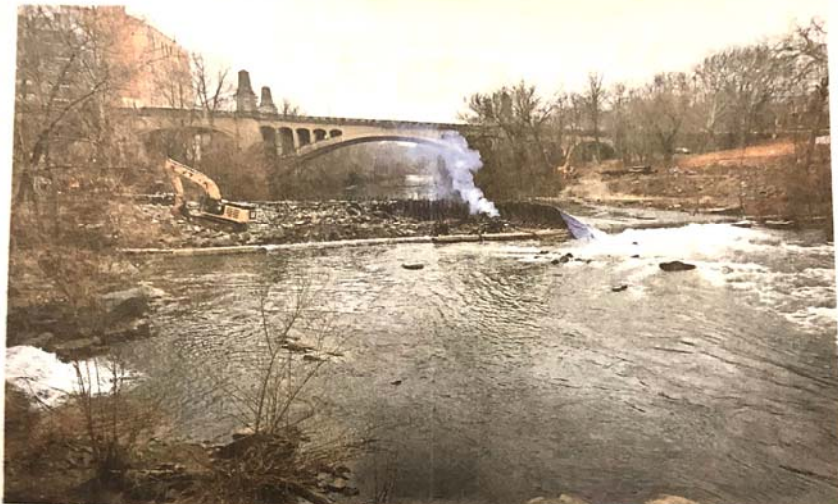
Crews are relocating a water main under Brandywine Creek as they remove a dam that has been blocking fish passage for 200 years. PHOTOS BY JENNIFER CORBETT/THE NEWS JOURNAL
