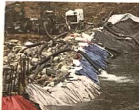
Removal of the dam is part of the work that is underway on the Brandywine River in Wilmington to restore the waterway to its historic roots.
