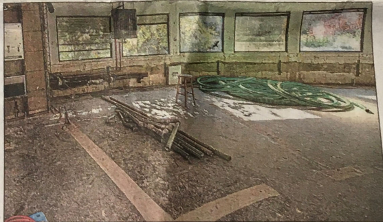
Floodwaters filled the lower level to the ceiling and damaged all 10 buildings. Above, the ground-floor museum offices. JOSE F. MORENO / Staff
