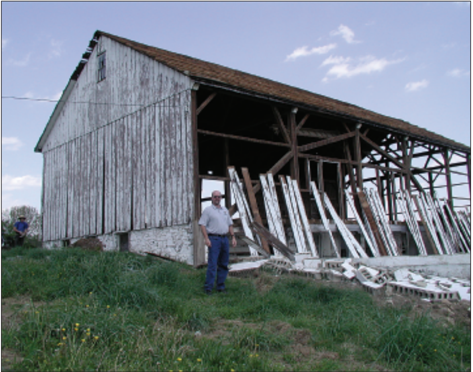
Figure 12. Koelig Farm barn before construction of Newark Reservoir in April 2002. In the foreground is lifelong Newark resident Martin Wollaston of the Water Resources Agency. (source: G. J. Kauffman, 2002)
