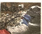
Removal of the dam is part of the work that is underway on the Brandywine River in Wilmington to restore the waterway to its historic roots.
