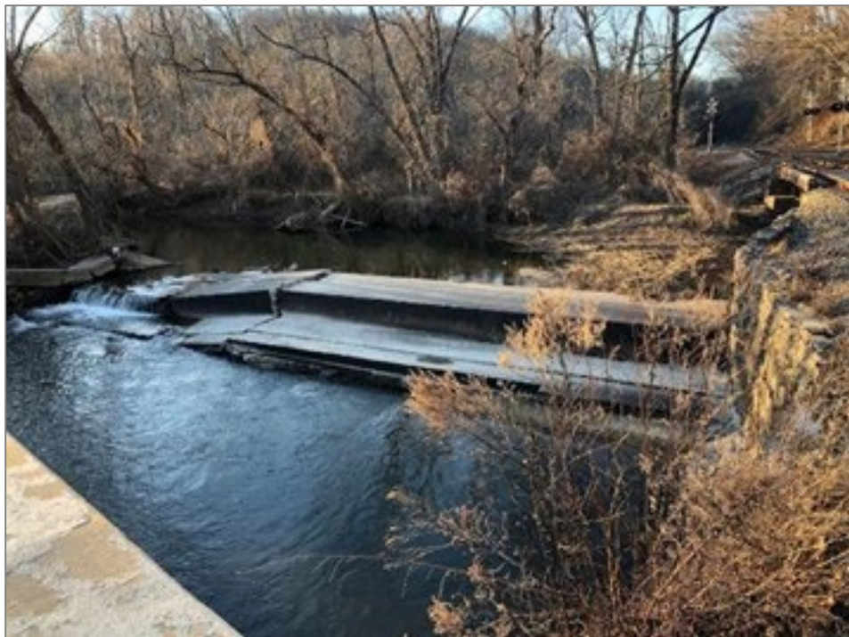
Sharpless Road dam failure along Red Clay Creek in Delaware
