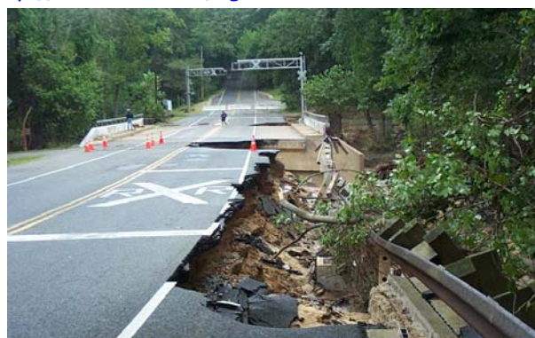
Damage to Faulkland Road and Bridge. Photo by John Talley
